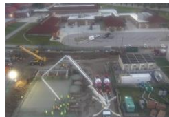
Chilled Water Capacity Enhancements
